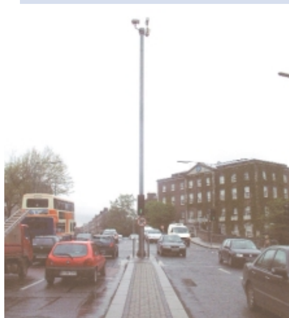
CCTV at traffic signal junction
