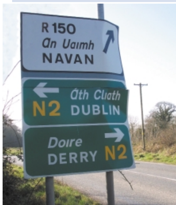
Signs damaged by HCV
